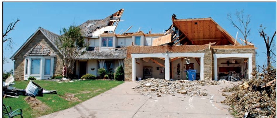
Figure 2-6: Example of a garage door failure that initiated progressive failure, including loss of the garage roof
